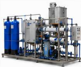
Water Treatment System (RO + UV + Filtration)
