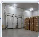
Cold Storage / Dispatch
